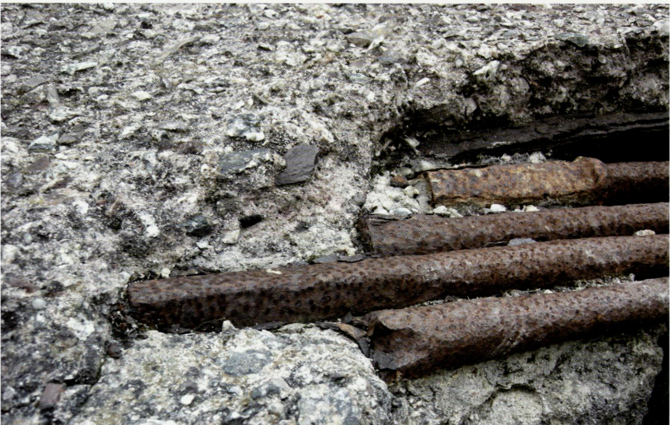
Old drill bits being re-used as reinforcement in the World War II air-raid shelter for workers at East Pool and Agar Mine. Photo: Martin Dixon
